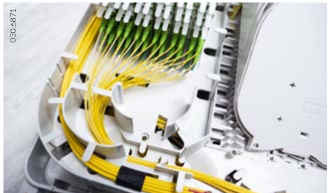
Safe laying of the fibers with gentle bending radius. Access to individual fibers is always guaranteed.
