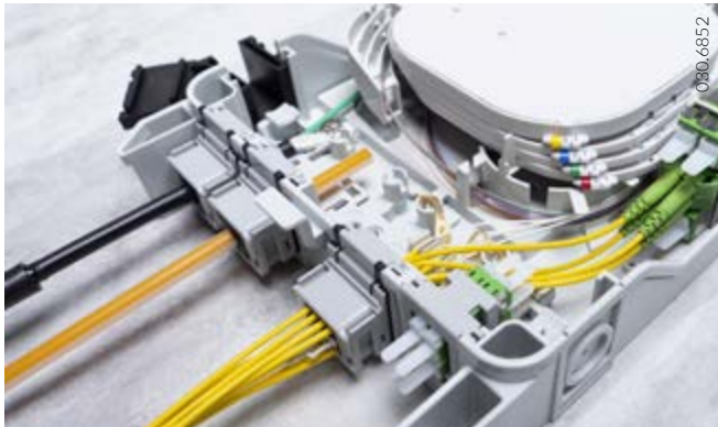
Cable entries on four sides and the rear (OTO application).
